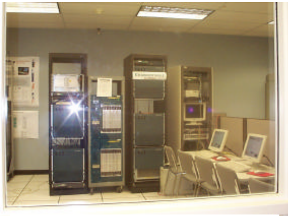
(a) Equipment Rack in the VINTLab.
